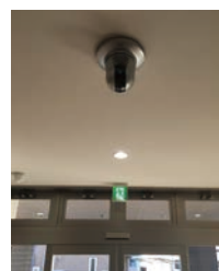
Security camera system for protecting facility users
