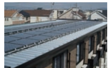
Photovoltaic power generation system
